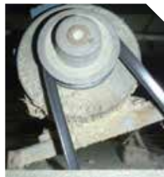
Figure 2 Incorrect fan belt sitting low in the pulley.
