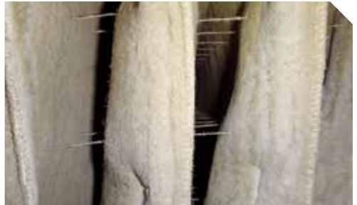
Figure 1 Air filters need to be checked and replaced regularly.
