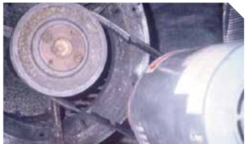
Figure 2 Fan belts should be checked regularly and replaced as necessary – this belt is not fit for use.
